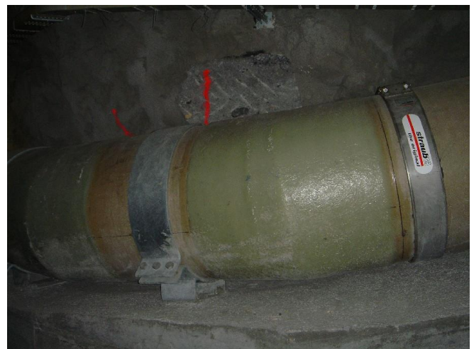
Anchoring points as retainer for traction- and crack forces within a bend.
