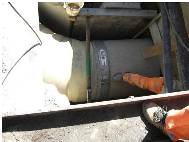
Picture: upon Direct connection between existing asbestos Tube DN 800mm with HOBAS tube DN 800mm
